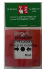
Evacuation / fire alarm button
