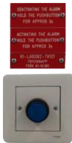
Figure 2. Spill / local warning button
