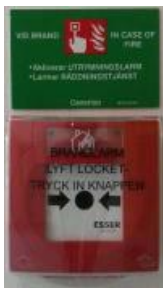
Figure 1. Evacuation/fire alarm button
